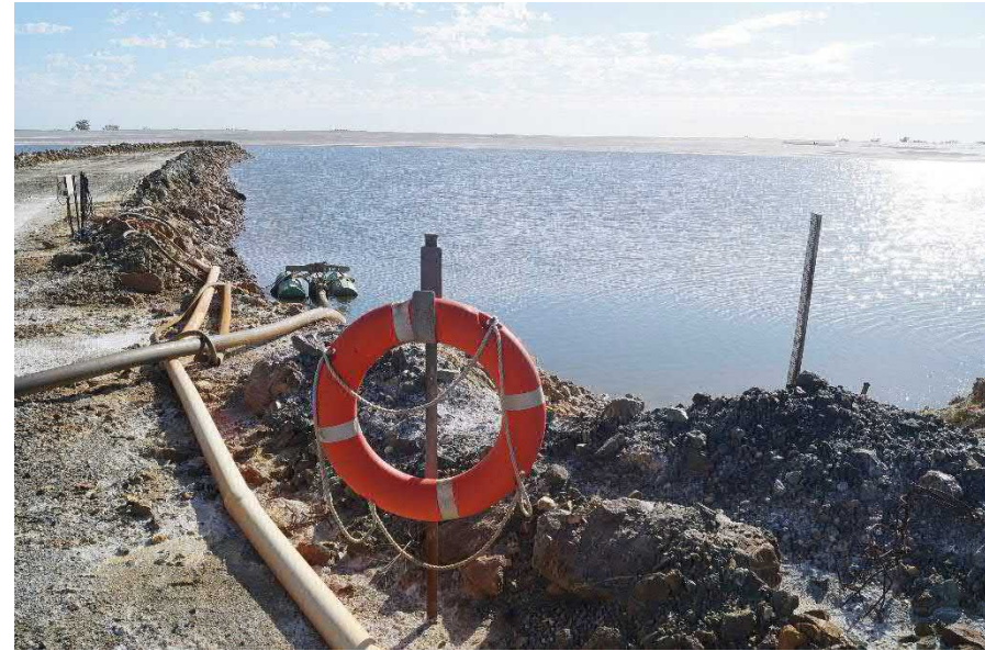
Floating water recovery pump and safety ring (17/2/2022)
