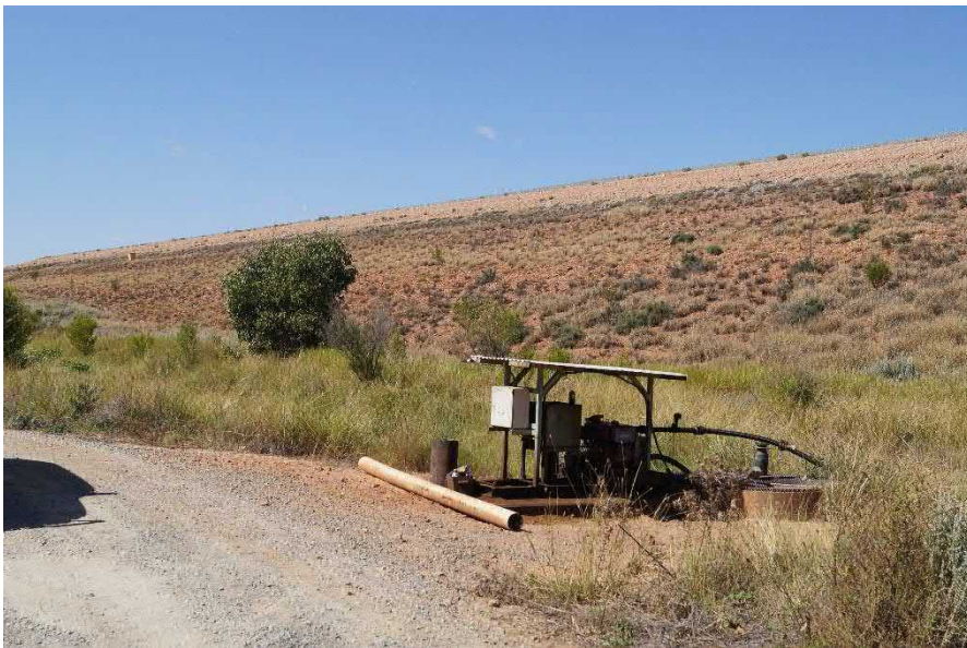
Underdrainage water recovery sump and pump (17/2/2022)
