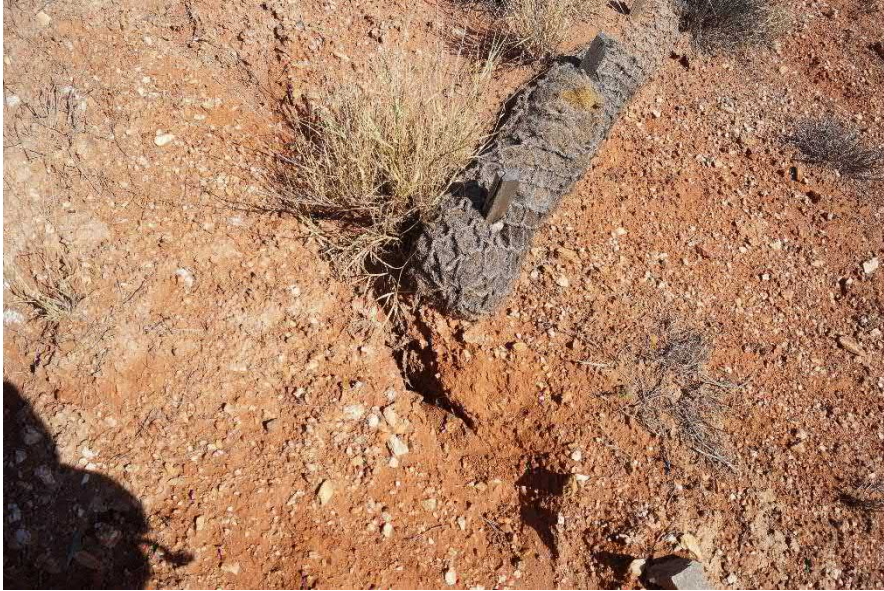
Scouring around an erosion control feature (17/2/2022)
