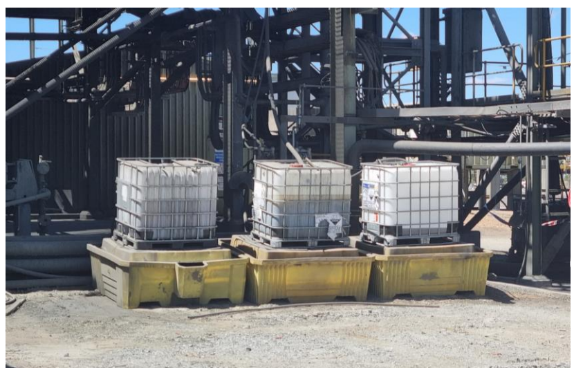
Photo 4 and 5: IBCs kept in self-bunded container or with dedicated bunding
