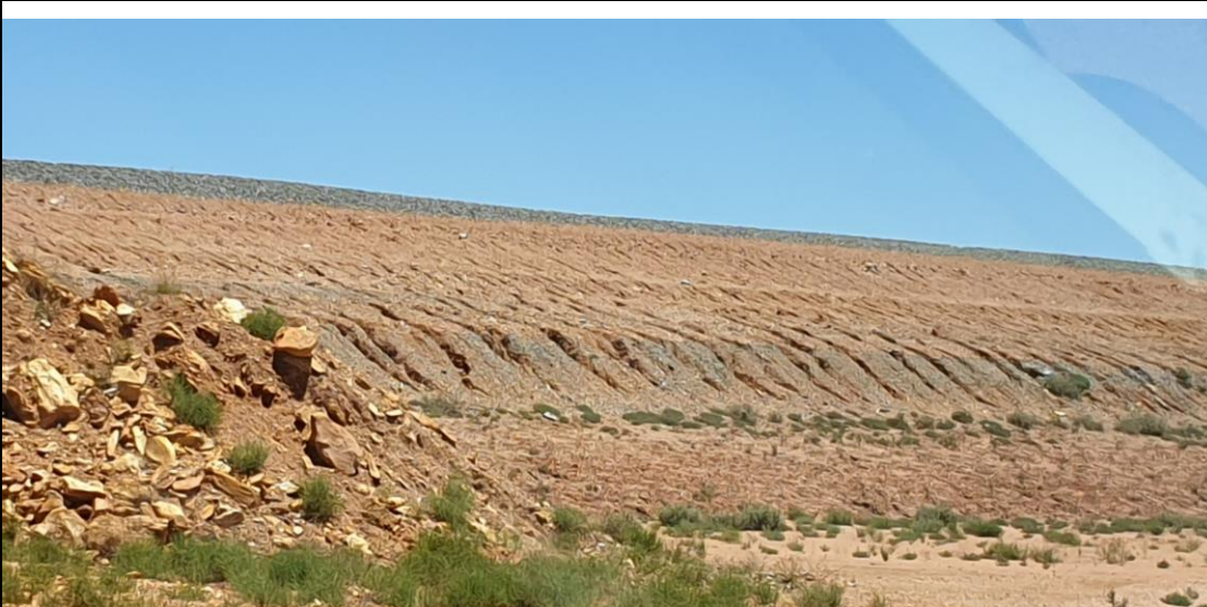
Photo 9: Localised erosion on the northern side wall of TSF embankment (Observation 1)
