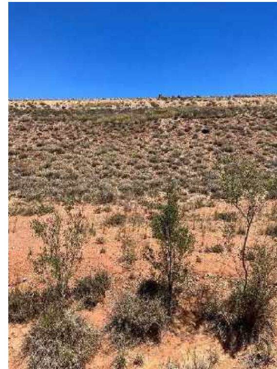
View of main embankment at piezometer PZH005 location. There are no signs of seepage.
