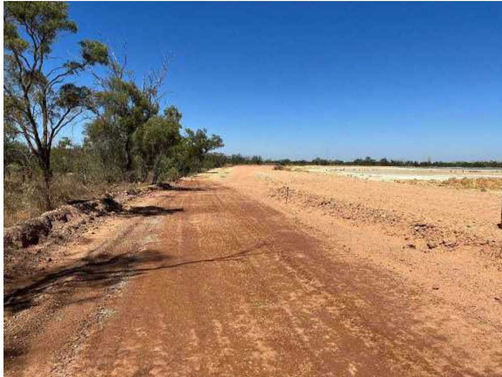
View along the southern side of TD1 showing new embankment looking west.
