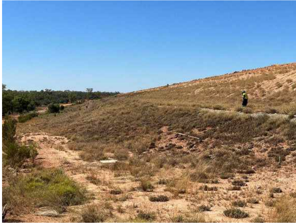
View from north east corner of main embankment looking south note vegetation cover.
