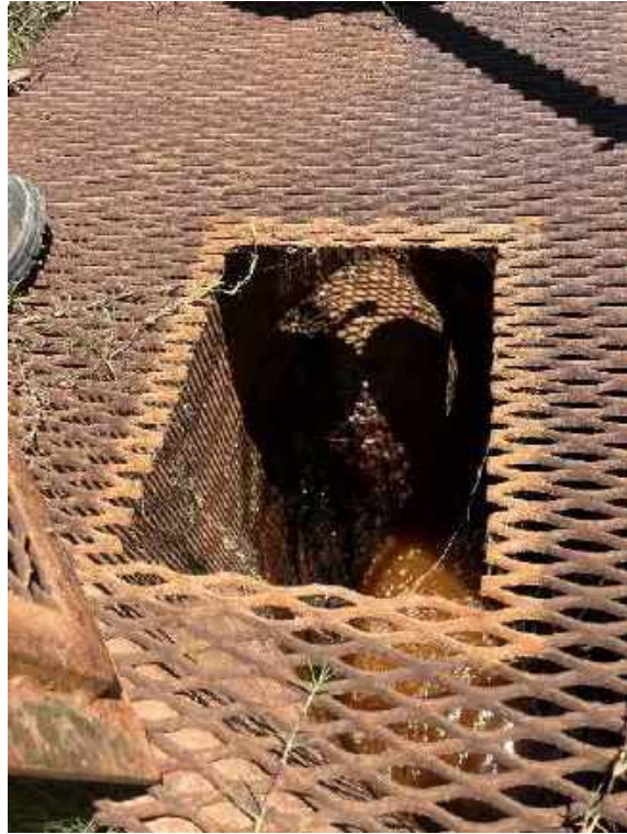
Underdrainage water flowing into sump for return to the process plant.
