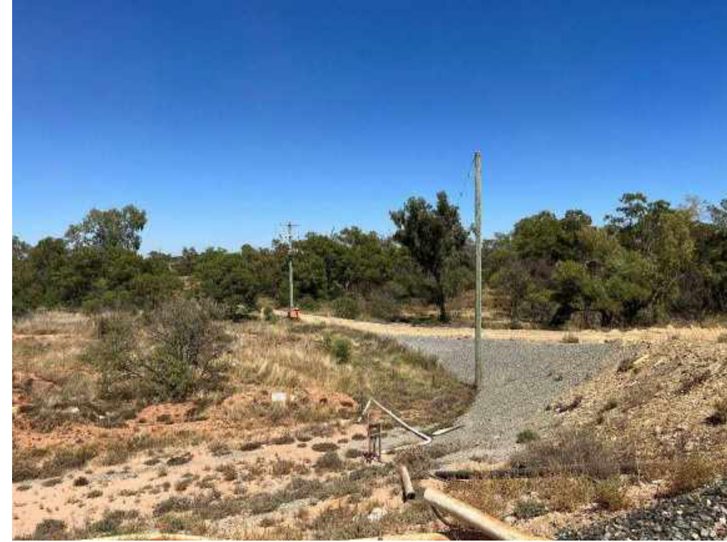
View from ramp on TD1 looking west. The rig in the background is working on a new vent riser.
