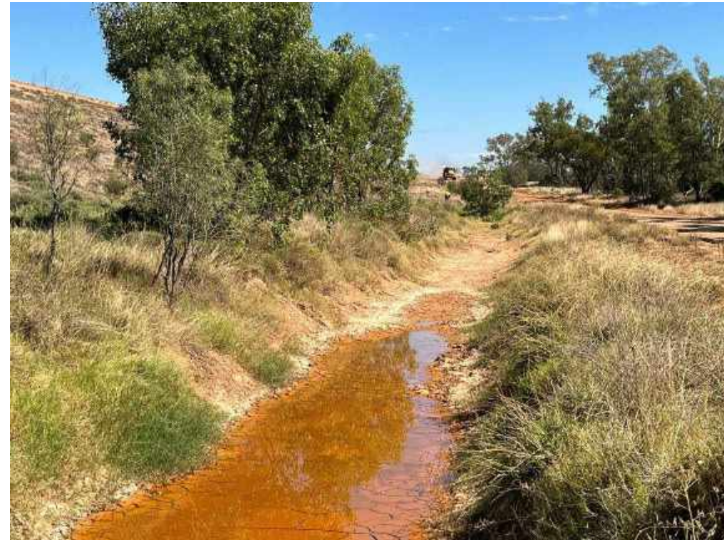
View looking north from sump, note water in drain adjacent sump. Pondered water cannot flow into sump.
