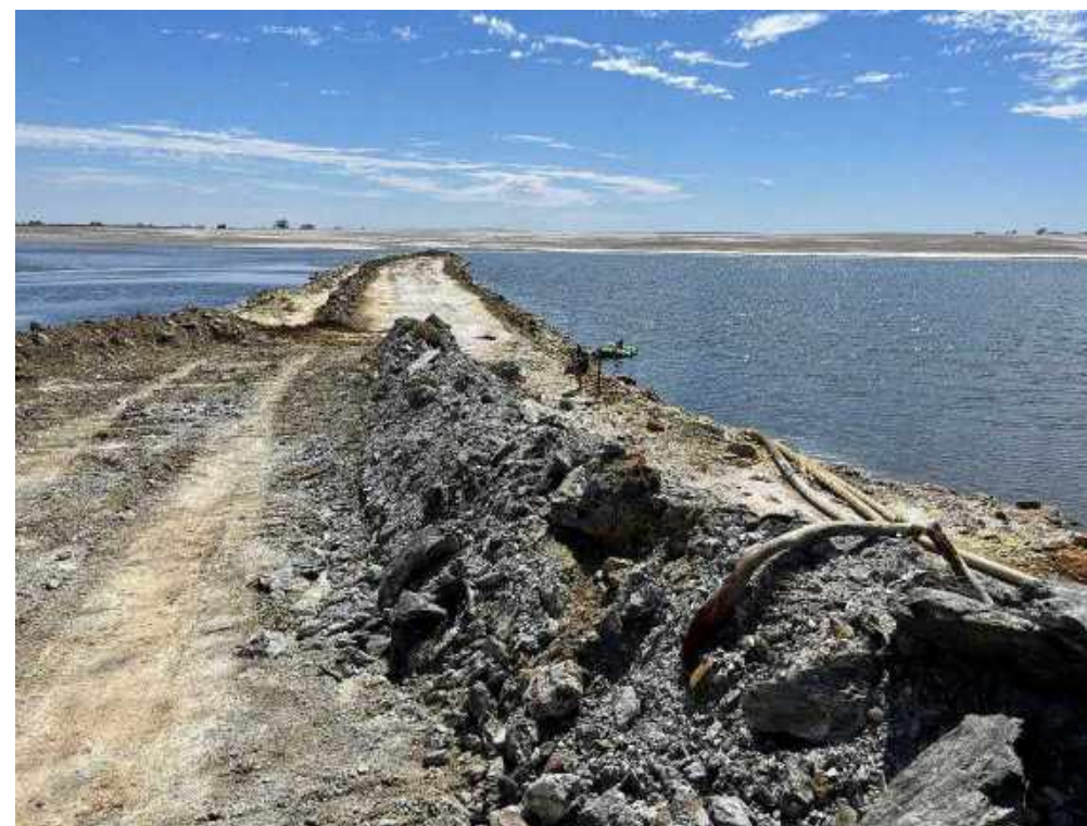
View along decant accessway, note water recovery pump in centre of photo.
