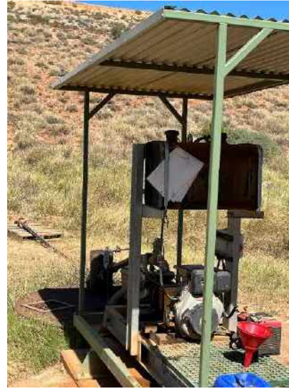
Underdrainage water recovery sump and pump.
