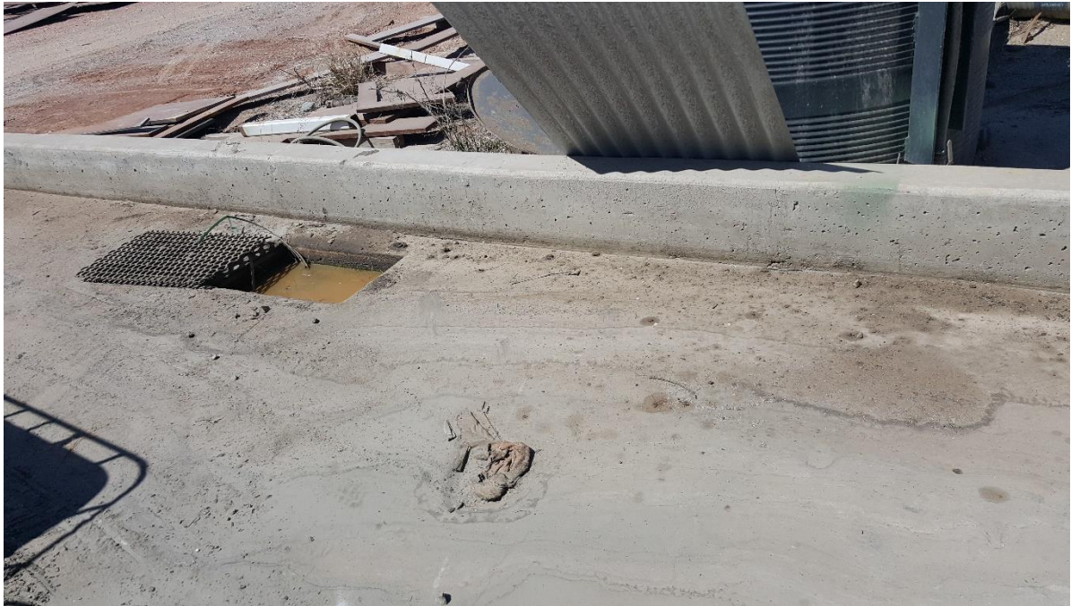
Drain within bunded area
