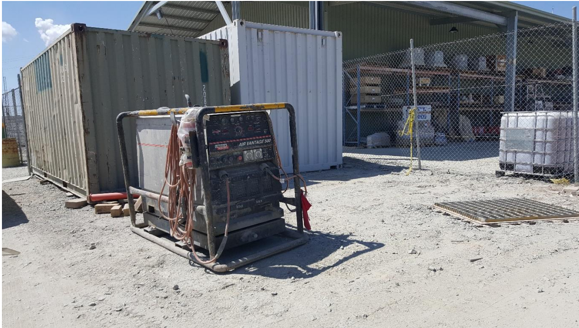
Placement of generator without bunding or pad
