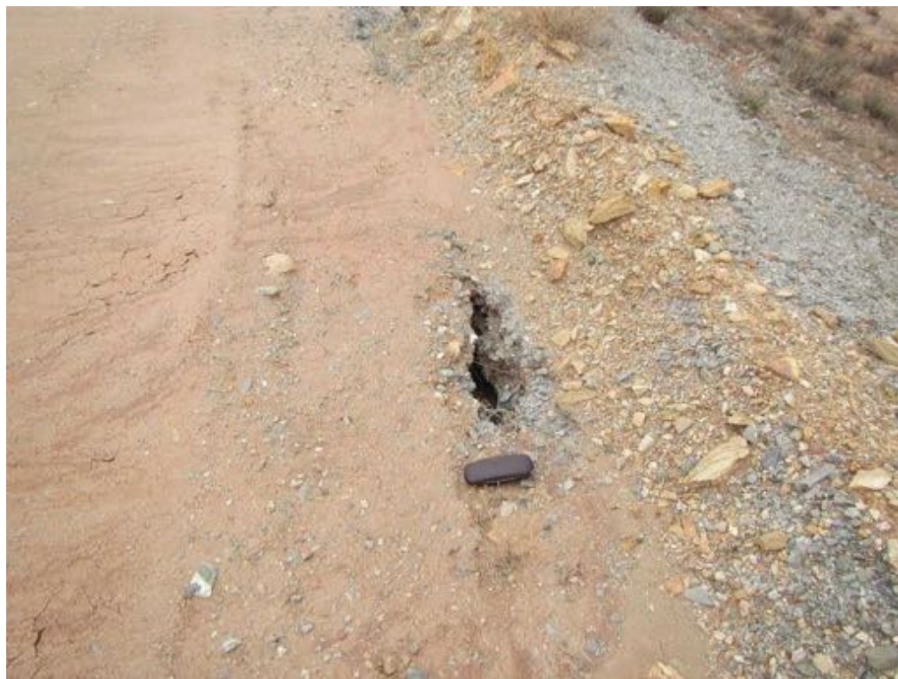
Piping crack northern end of intermediate berm, .
