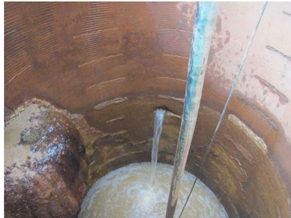
Sump receiving toe drain water southern side and underdrainage inflow.
