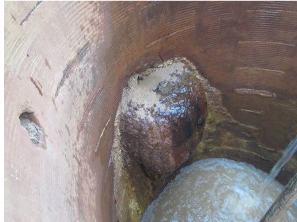
Underdrainage recovery sump still receiving underdrainage flow after 15 years of operation.
